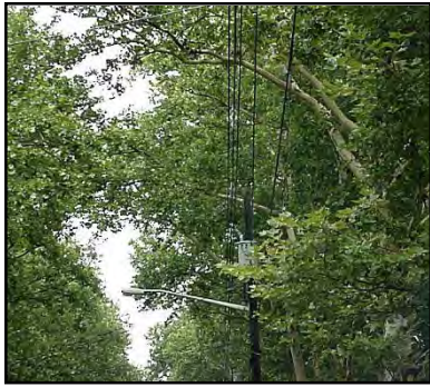
Directional pruning can train the canopy to grow away from or over conductors.
