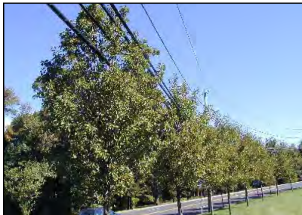
A formula for failure: Misplaced trees = loss of aesthetics + increased maintenance concerns.
